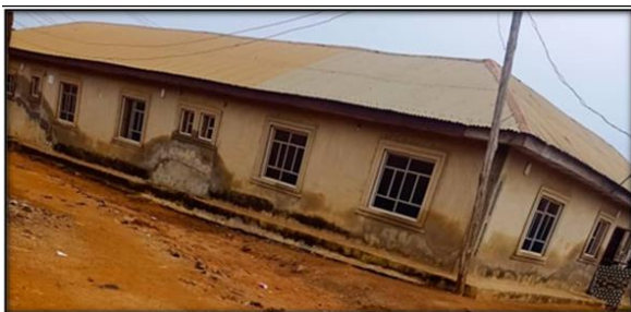
Figure 2: Example of wall Dampness.
