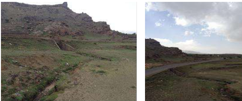
Figure 13a: Water Erosion in culvert Outlet Located in Plain Slope
