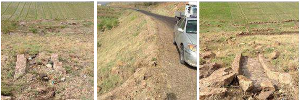
Figure 10b: Blocked Roadside Spillways in Shoulders
