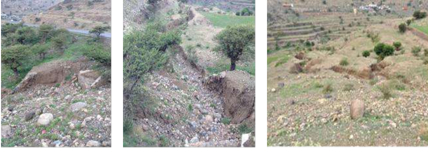
Figure 13b: Water Erosion in Culvert Outlet Located in Steep Slope
