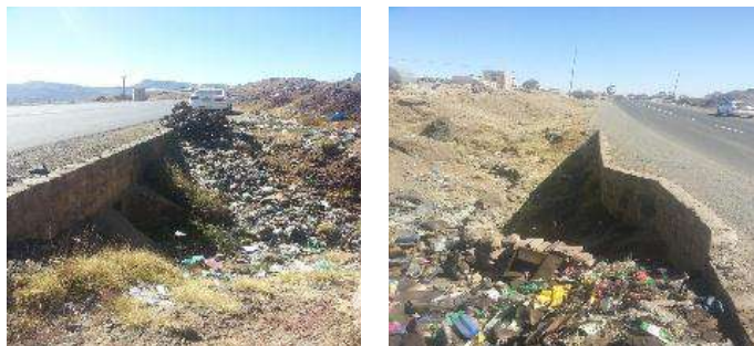
Figure 14b: Water Ponding near the Culverts due to Poor Maintenance
