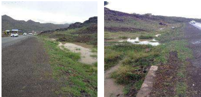
Figure 14a: Water Ponding at Side Drain due to Poor Maintenance
